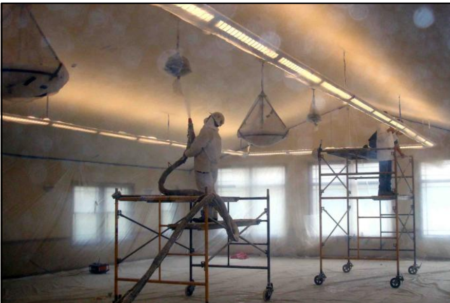
A crew from Stony Creek Services applies "SonaKret" Acoustic Finish in the dining room. The material was applied in 5 layers and hand troweled. It offers a 0.75 Noise Reduction Coefficient (0 = no absorption; 1 = complete absorption).
